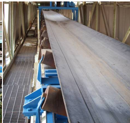
Conveyor from stockpile
