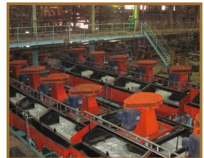
Flotation cells commissioning
