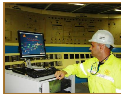
New concentrator control system (with old in background)
