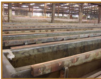
Completed electrowinning cells
